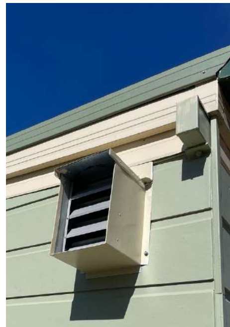
New Air Vent for ETG room
